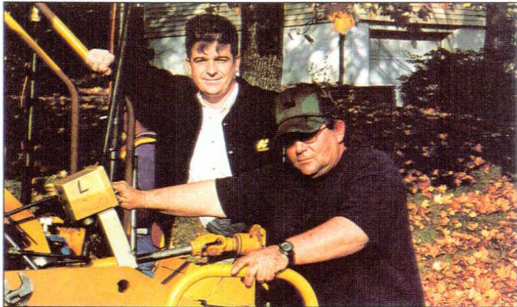
Jim Cleary instructs Dave Holton, Schifano paving foreman, on use of the sonic control.
