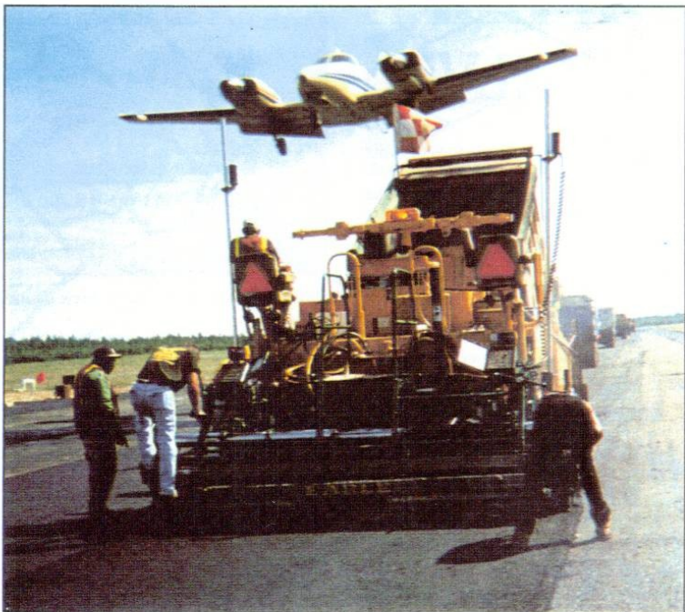
Grade control system used by Earle Asphalt at the Robert J. Miller Airport.
